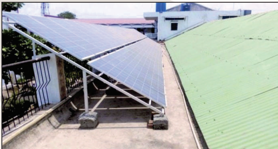
Fig.1 Erected solar panel at rooftop.
